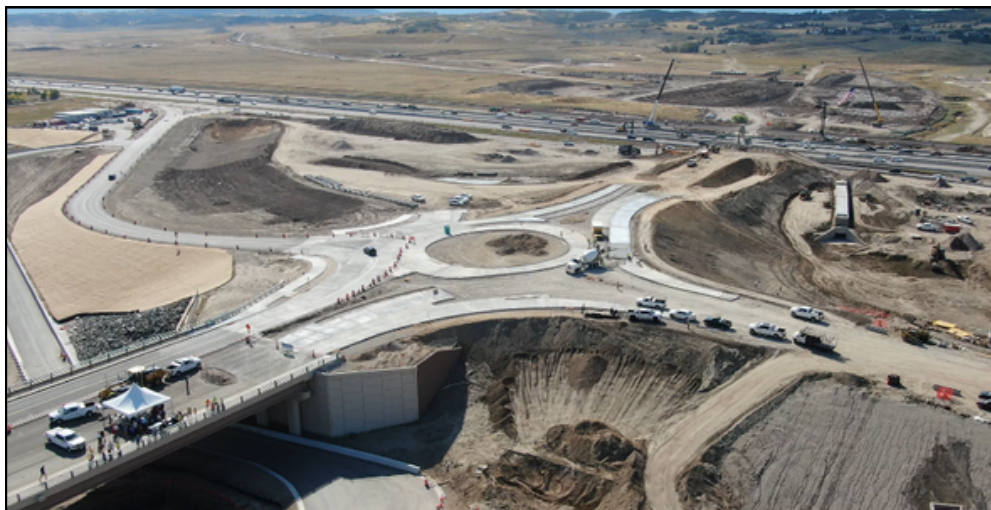
Aerial photo of the Crystal Valley interchange project area taken September 26. Photo courtesy of Town of Castle Rock.
