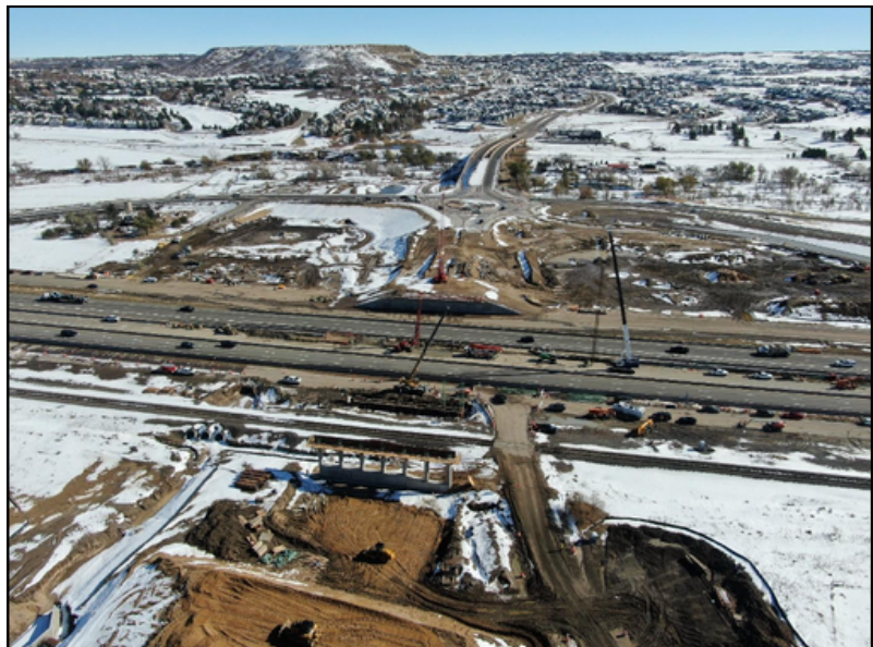
Aerial view of the project area in November, featuring foundation work for the future bridge over I-25, and the new portion of the East Frontage Road and roundabout intersection at Crystal Valley Parkway.
