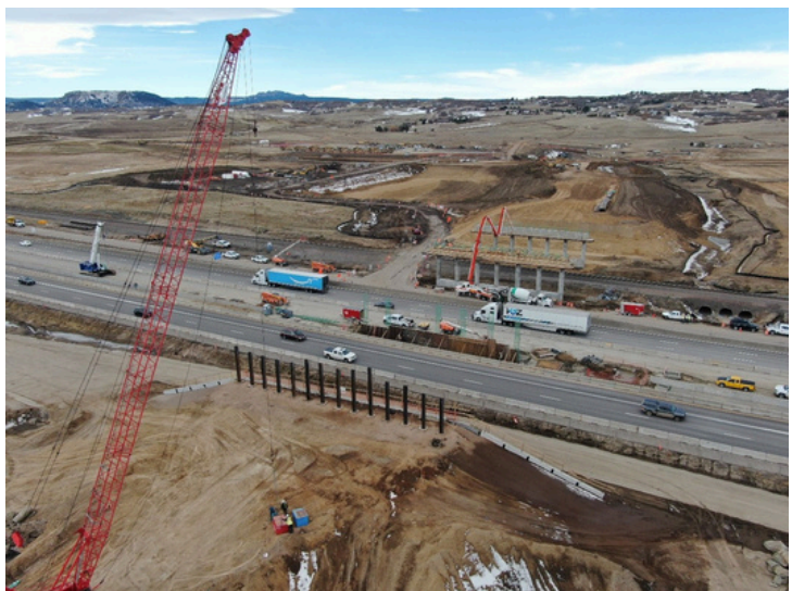
Ongoing I-25 bridge work. Photo taken December 2024. Photo used with permission of Town of Castle Rock.
